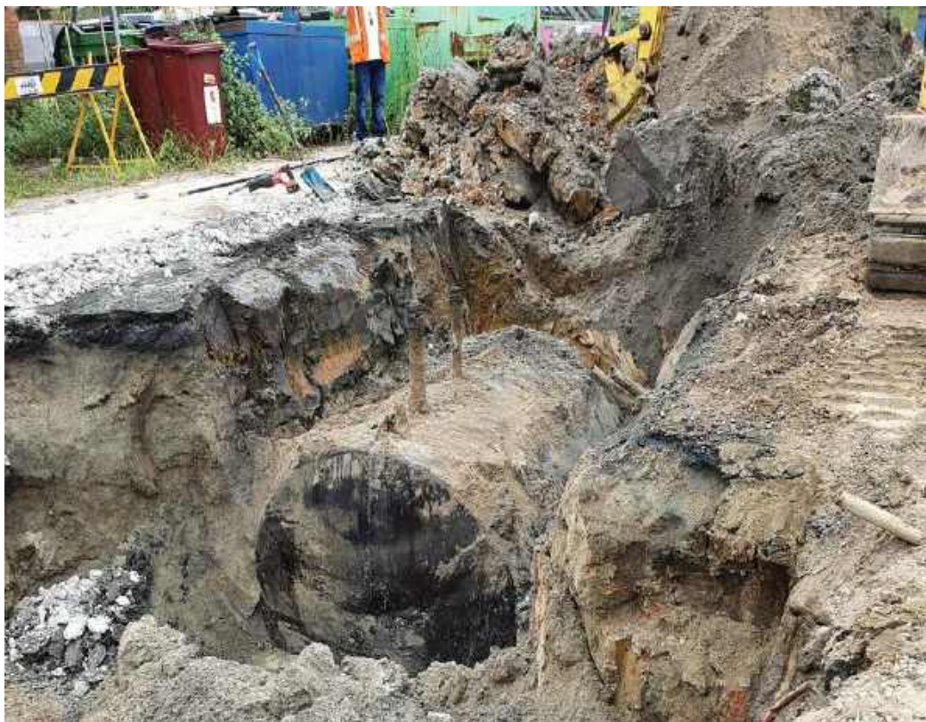
PHOTOGRAPH 2 Black staining on northern wall adjacent Tank 3.
